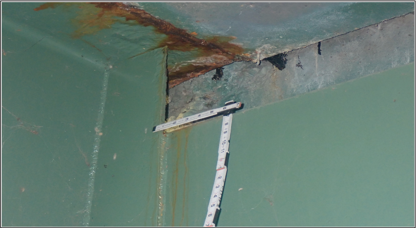
19 WEST ABUTMENT BACKWALL DEEP SPALL BEHIND GIRDER 1
