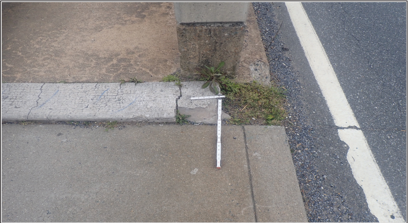
7 SOUTH SIDEWALK DEEP SPALLS AT EAST END
