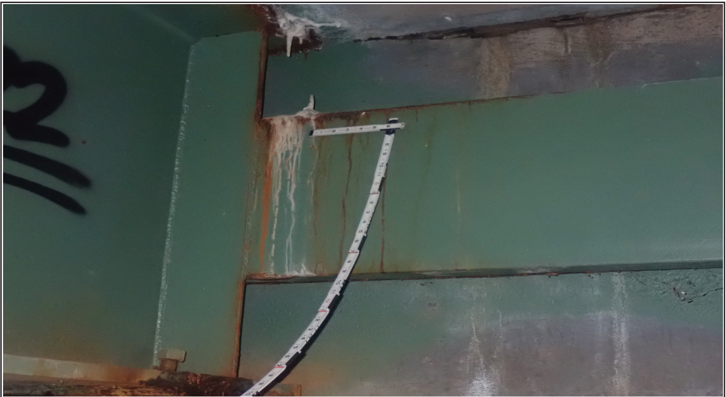
16 DIAPHRAGM BAY 2 CORROSIONN w/LOSS OF SECTION OVER WEST ABUTMENT
