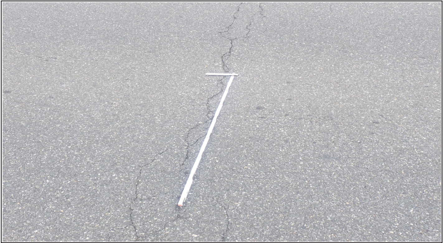
11 AC OVERLAY WIDE CRACKS IN WESTBOUND LANE
