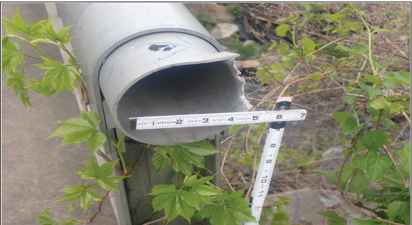
8 SOUTH METAL RAIL TEAR / DAMAGE WEST END
