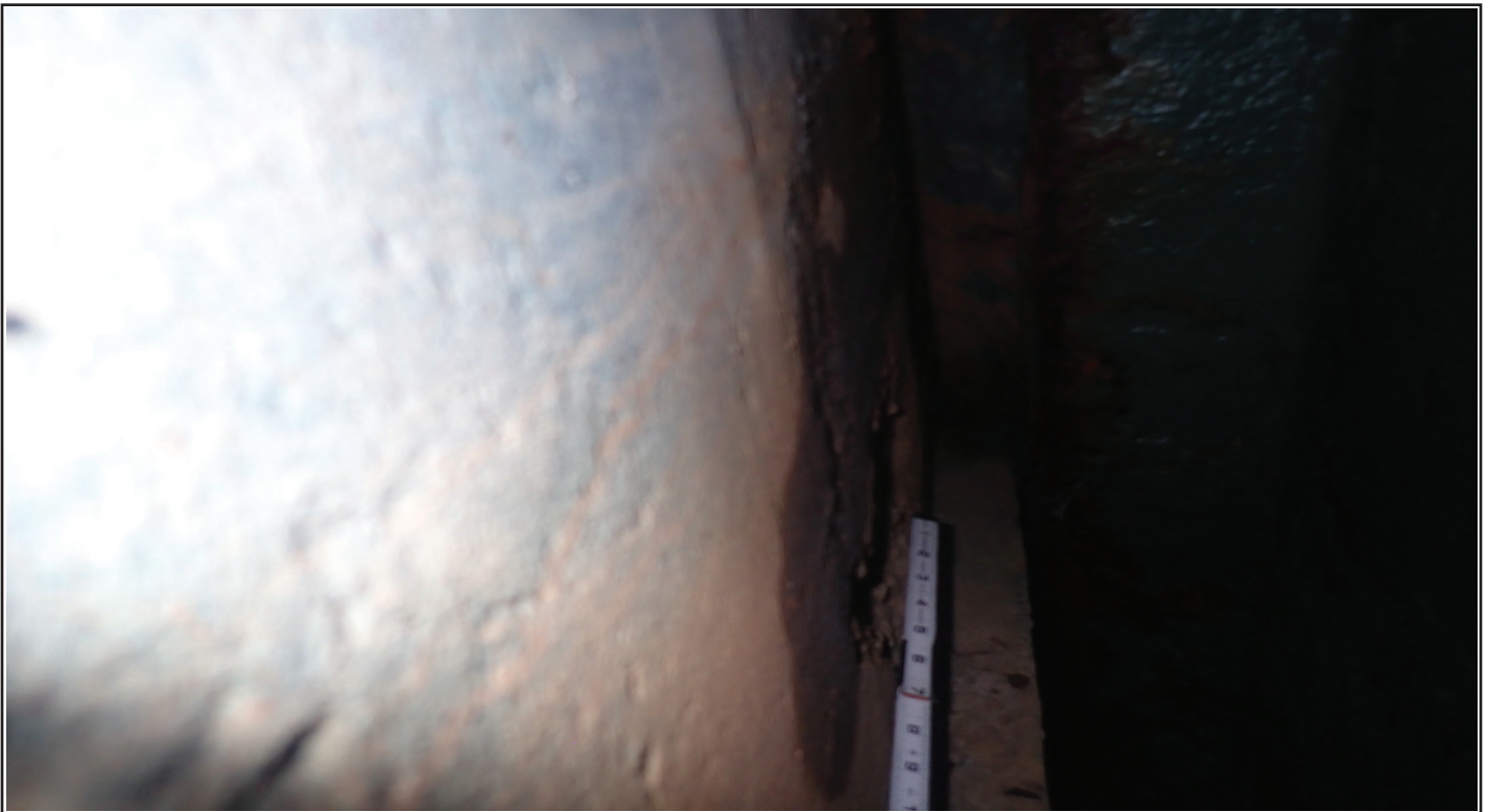
20 ARCH DEEP SPALL SOUTH FACE ADJACENT TO GIRDER
