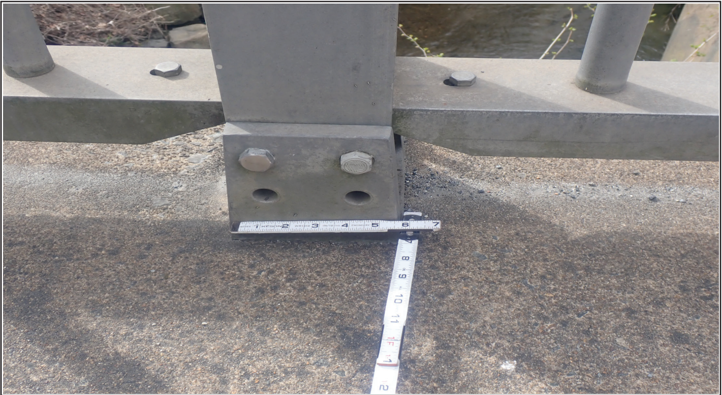
9 SOUTH METAL MISSING CONNECTION AT POST 2 FROM WEST
