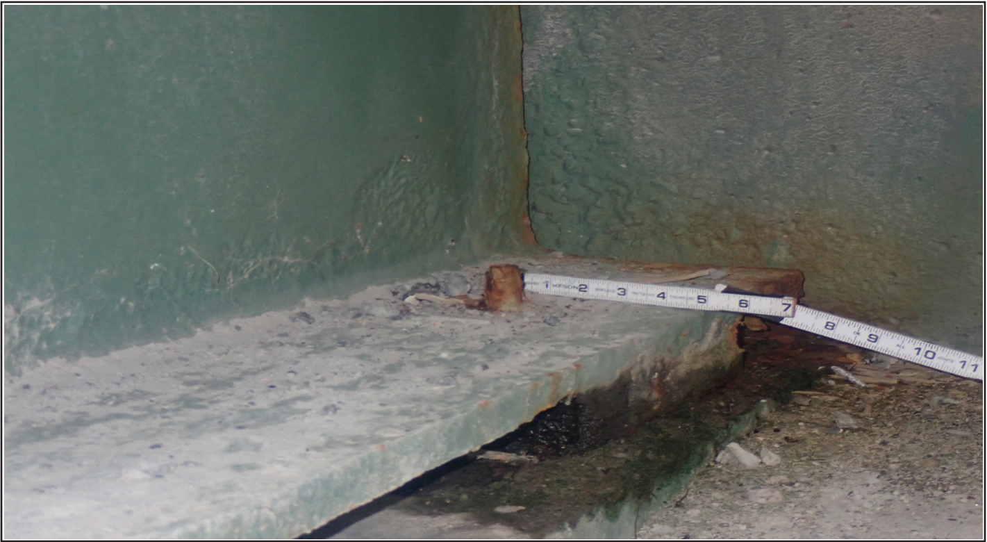
13 FIXED BEARING 1 OVER WEST ABUTMENT MISSING CONNECTION
