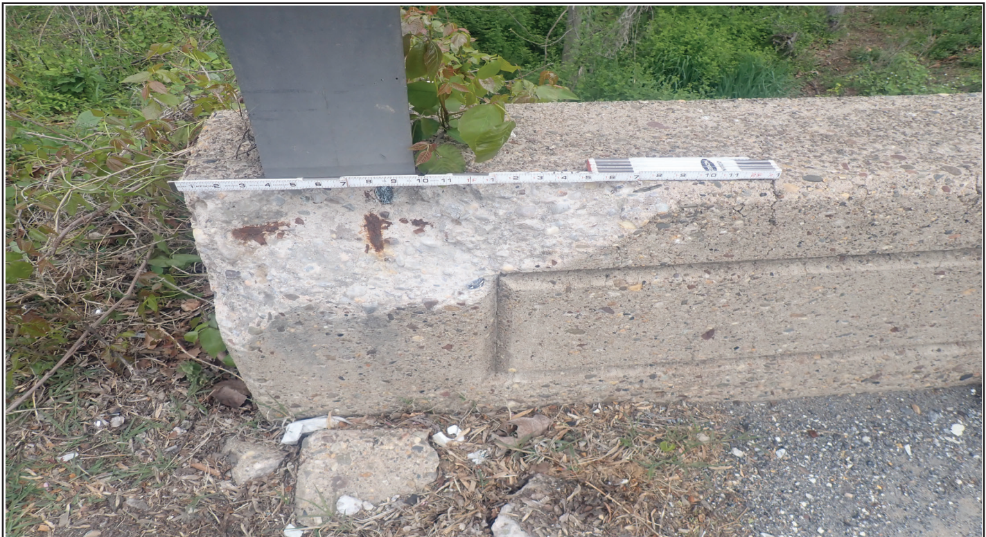
12 NORTH RAIL EXP BARS w/LOSS OF SECTION AT WEST END
