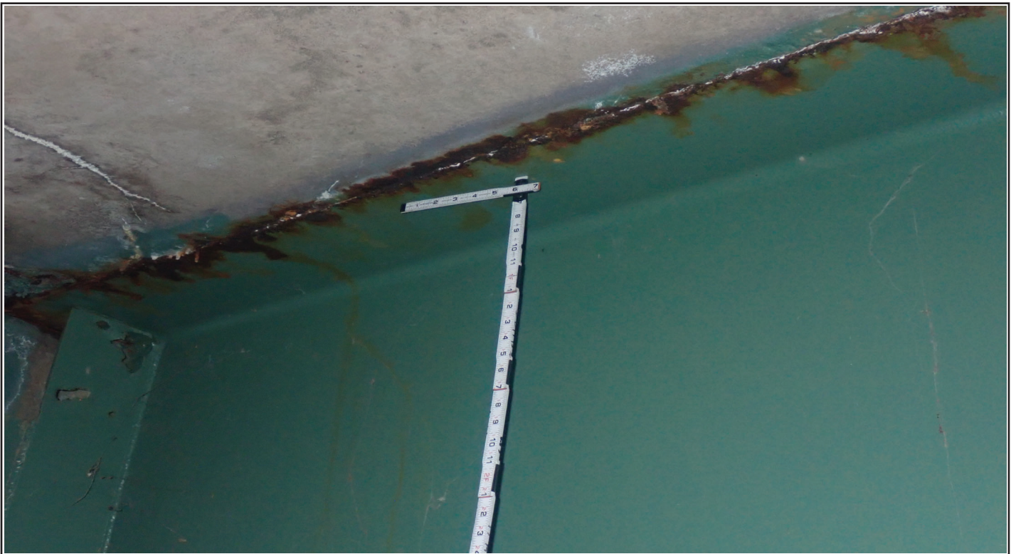
14 GIRDER 1 TOP FLANGE CORROSION w/LOSS OF SECTION OVER WEST ABUTMENT
