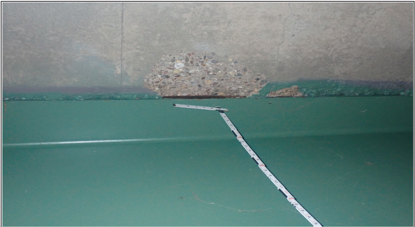
18 SOFFIT BAY 1 DEEP SPALL NEAR MID SPAN
