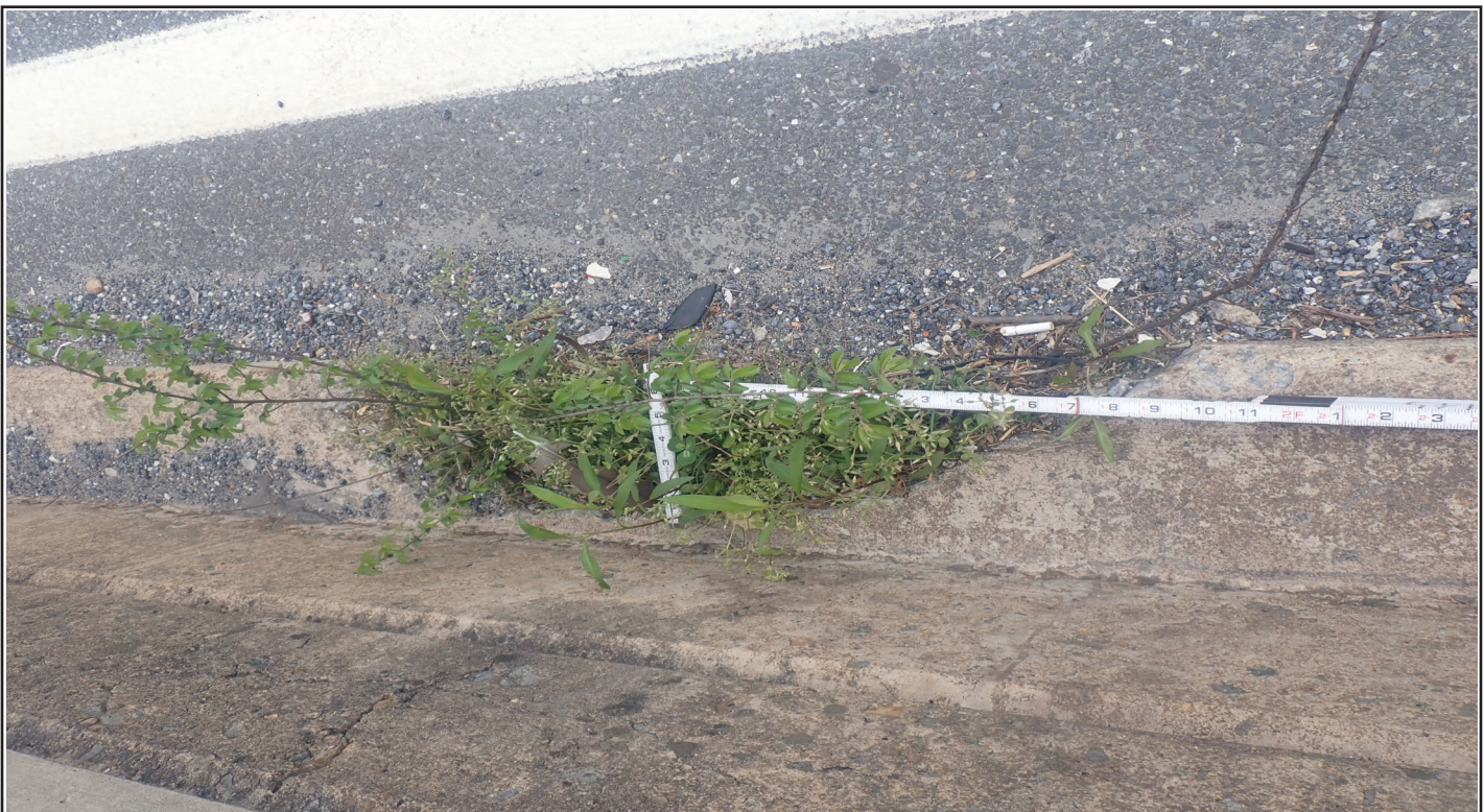
10 SOUTH RAIL DEEP SPALL NORTH FACE MID SPAN
