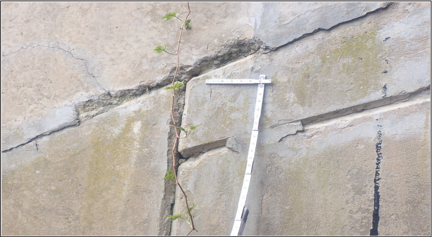
21 SOUTHWEST WINGWALL DEEP SPALL MID SPAN
