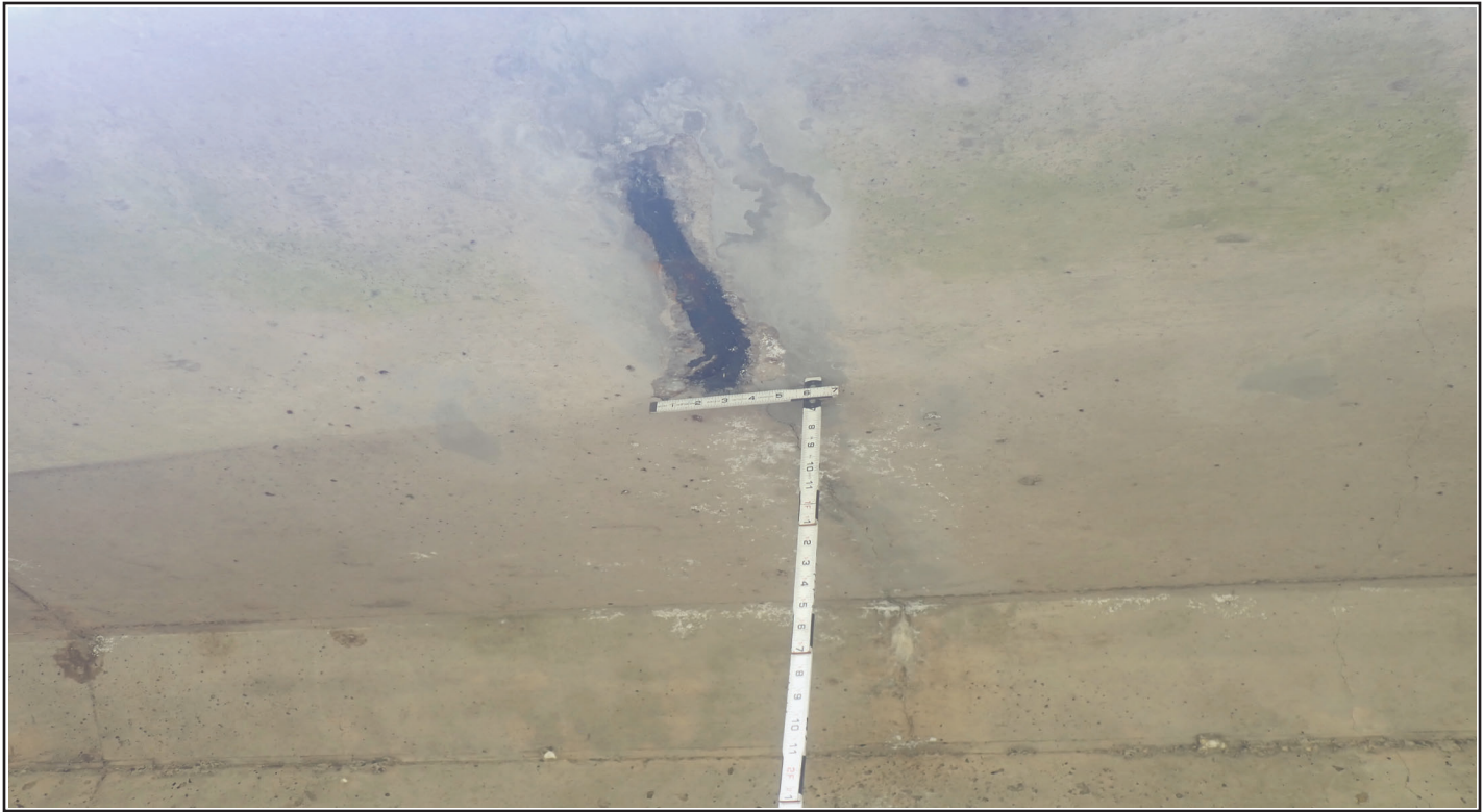
17 SOFFIT NORTH OVERHANG EXP BAR w/LOSS OF SECTON NEAR MID SPAN
